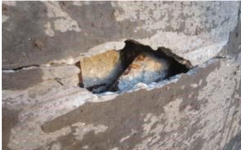
Figure 1. Expulsion of concrete due to infiltration of salt water.
