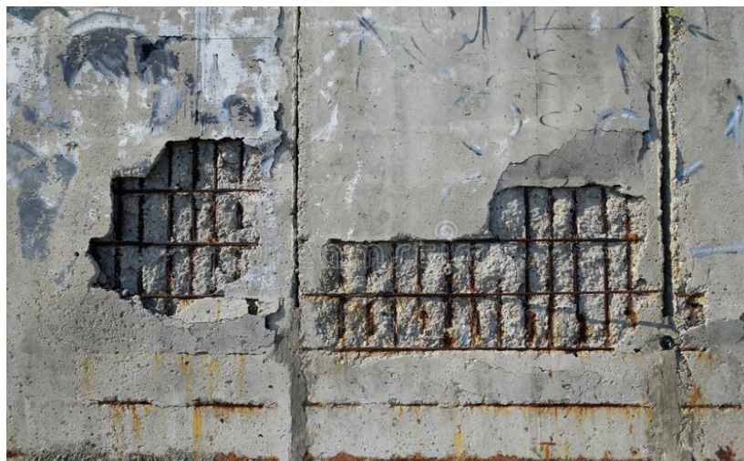
Figure 2. Due the corrosion process, the concrete coating can be removed, leaving the reinforcement unprotected.
